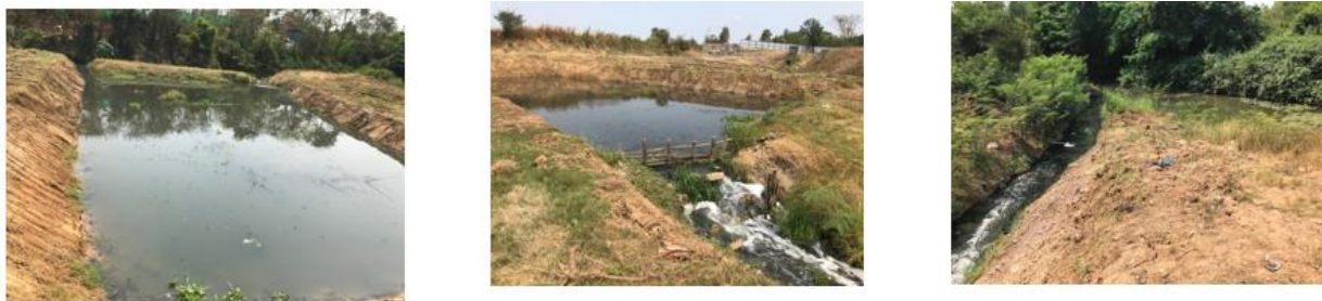
Figure 2: Constructed wetlands area developed by the municipality downstream of Aranyaprathet – after damage from annual flooding. Constructed wetland (left), plant and grass filtration (middle) and water flow to Phrom Hoad canal (right)
