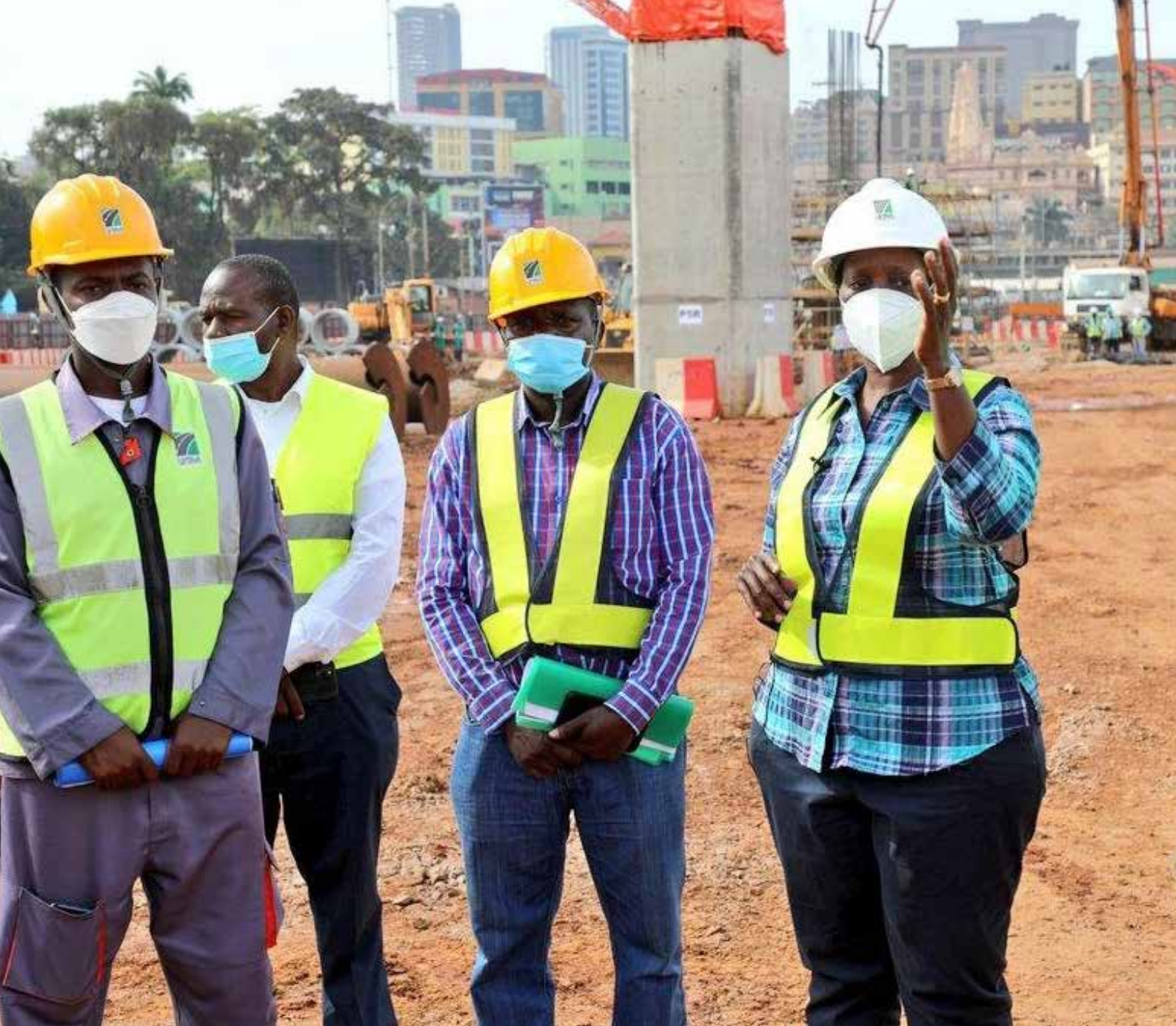
UNRA officials monitoring the progress of the Kampala Flyover Road Upgrading Project
