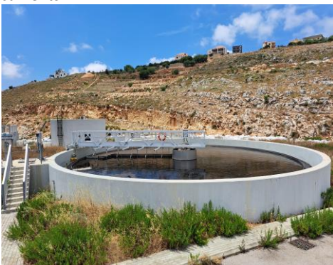
Tebnine Wastewater Treatment Plant
