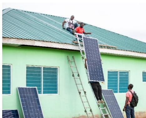
Left: Students at a Technical Training Institute are learning how to work on solar panels. The practical approach will help them being well equipped for the job as solar technician.
