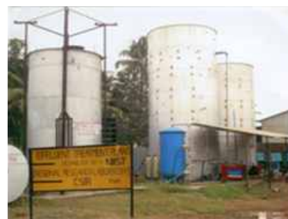
Effluent Treatment Plant
