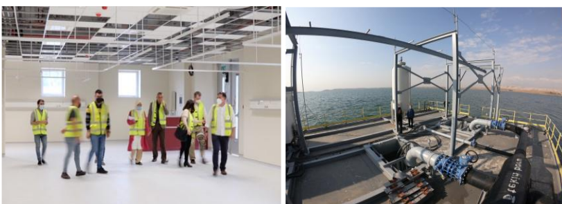
Photo left: Construction phase of the new Emergency Wing at the Azadi Teaching Hospital in Duhok city
