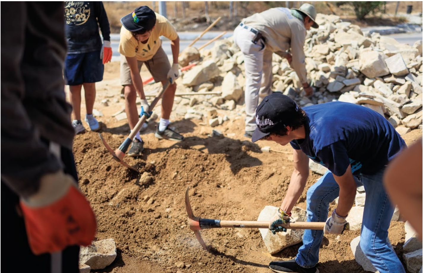
Clearing ground for the creation of a micro-basin ©GIZ México, Josafat de la Toba.
