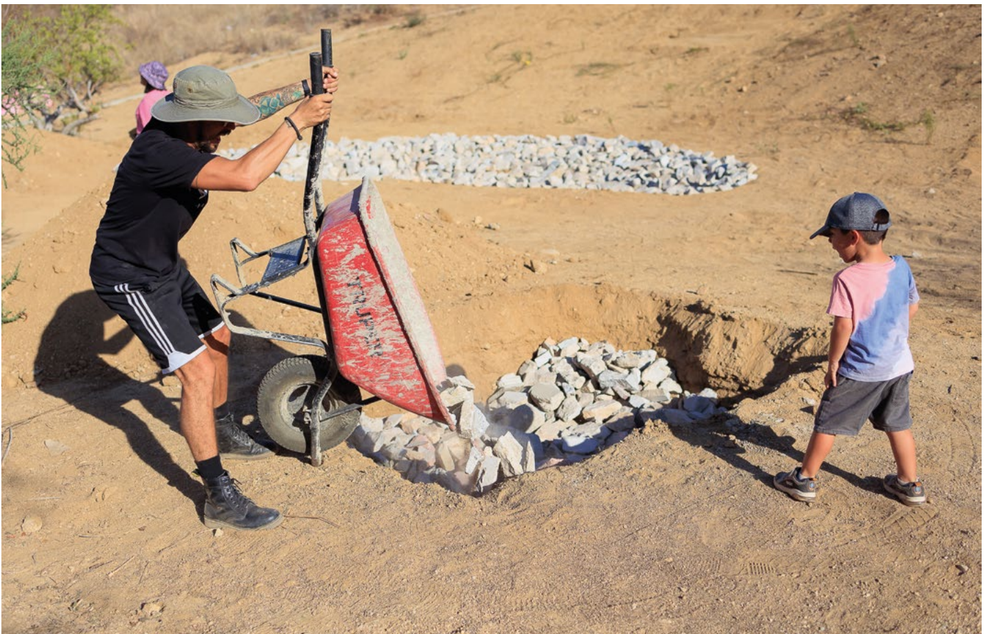
Community filling absorption well with material ©GIZ México, Josafat de la Toba.
