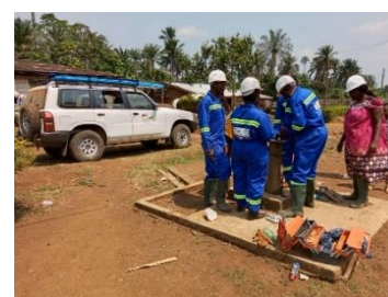
Practical training for council technical staff in the maintenance of a water point
