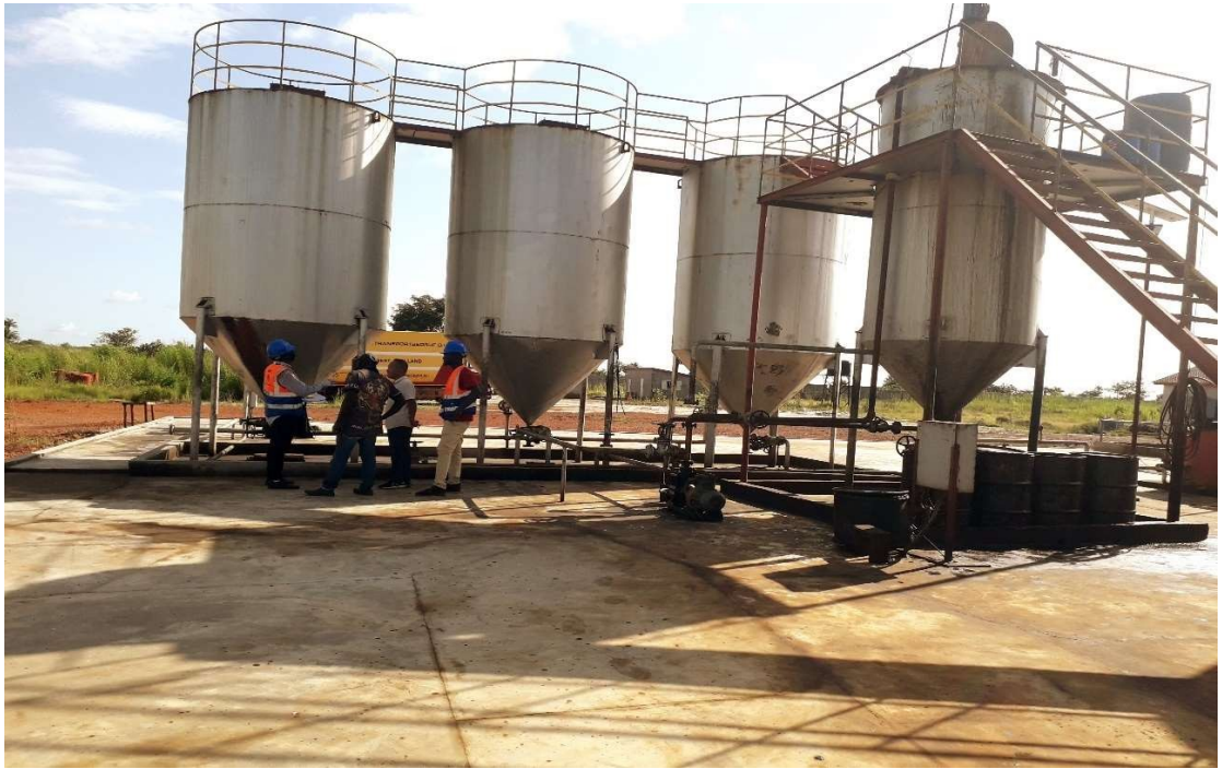
Image 23: Used oil processing line
