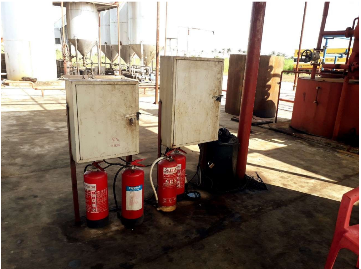
Image 23: Fire extinguishers at the Tanènè facility
