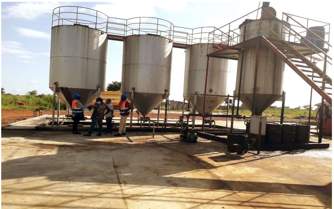
Image 23: Used oil processing line
