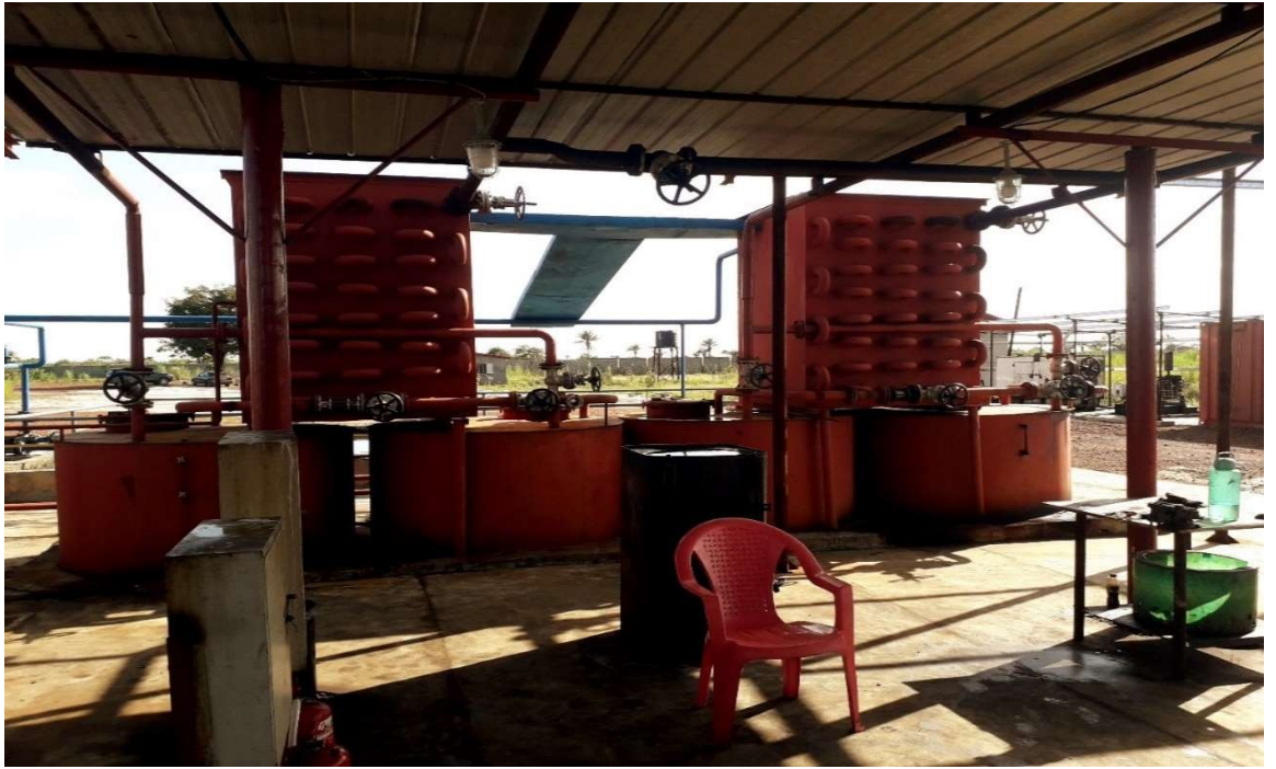
Image 24: The cooling system at the Tanènè waste oil recovery plant
