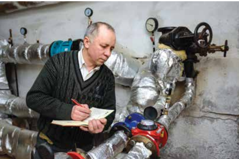
Energy manager of a hospital checks the radiators
