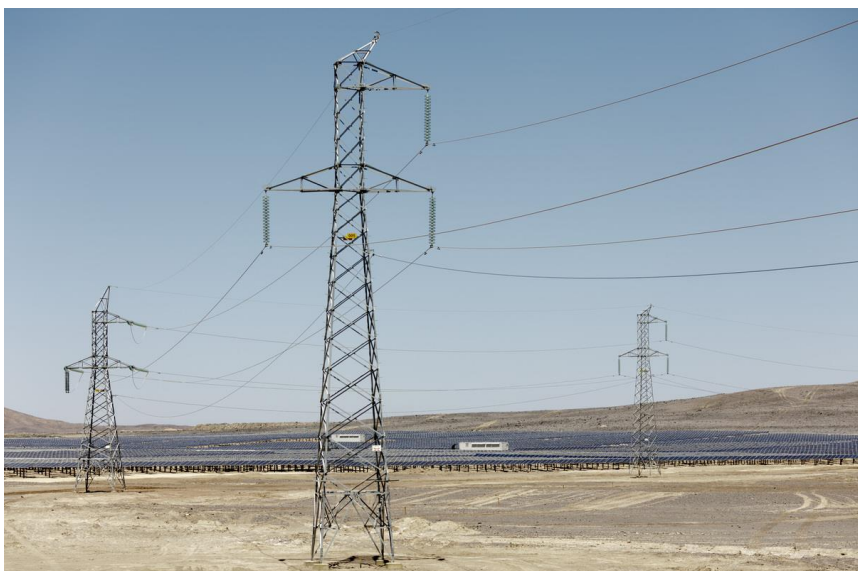
Electricity pylons in front of a large photovoltaic plant
