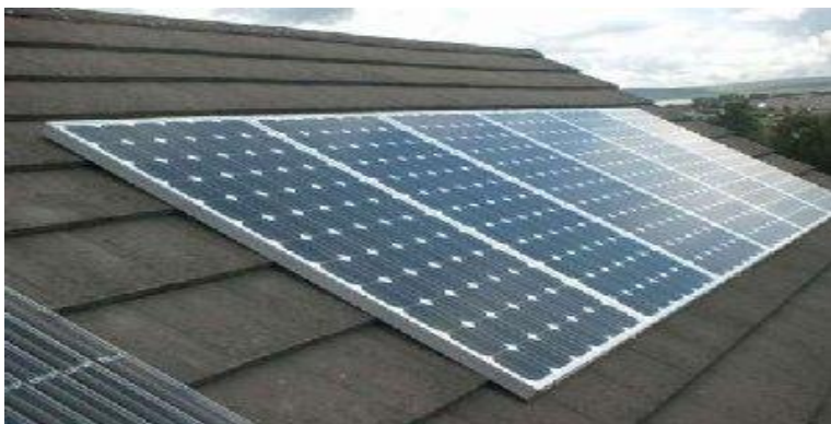
Figure-31: Rooftop PV installations
