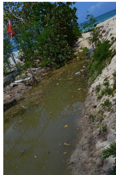
Drainage ditch, showing blocked sea outfall which prevents the flow of storm water. (2017)
