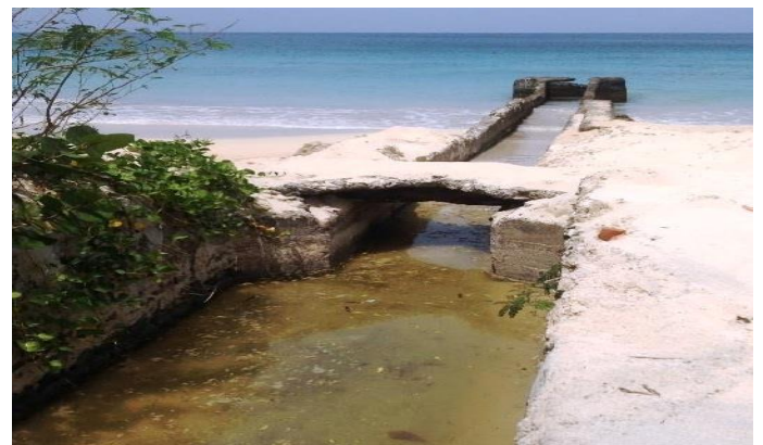
Derelict South Drainage of Grand Anse (2016)
