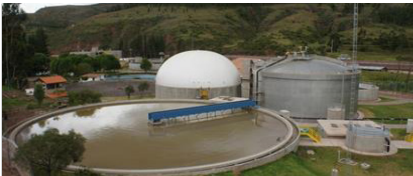
Biogas production in the wastewater treatment plant of Cusco.
