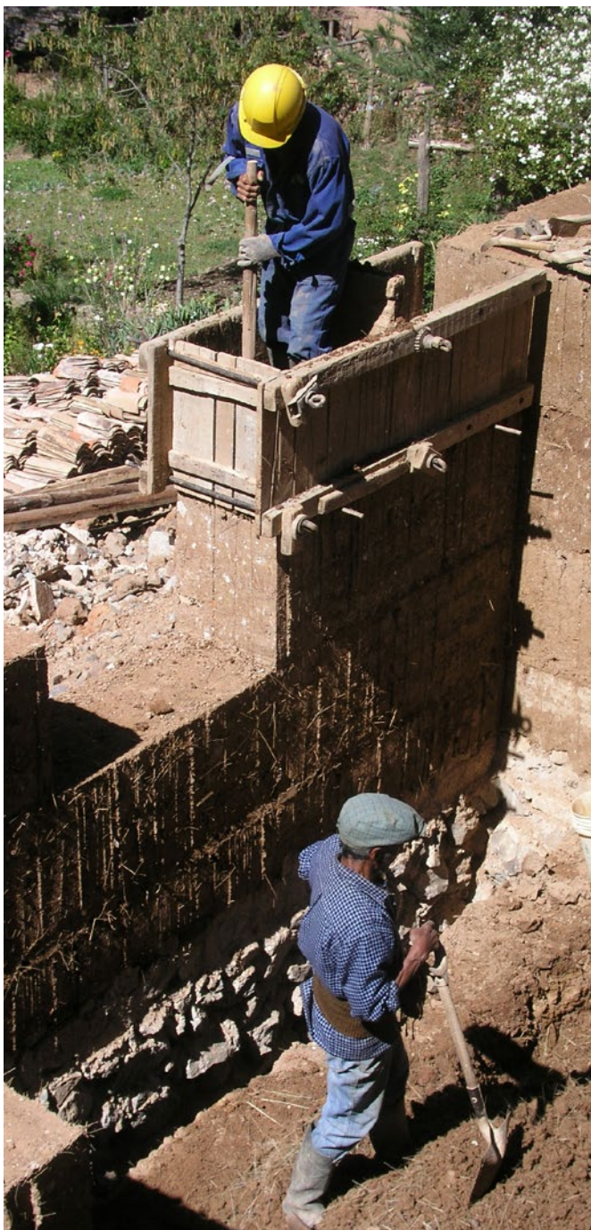
Rammed earth buildings in the Hacienda Santa Maria, Tarma, Junin, Pérou. Author: JYB Devot. https://commons.wikimedia.org/wiki/File:PiseP1010653mod.jpg
