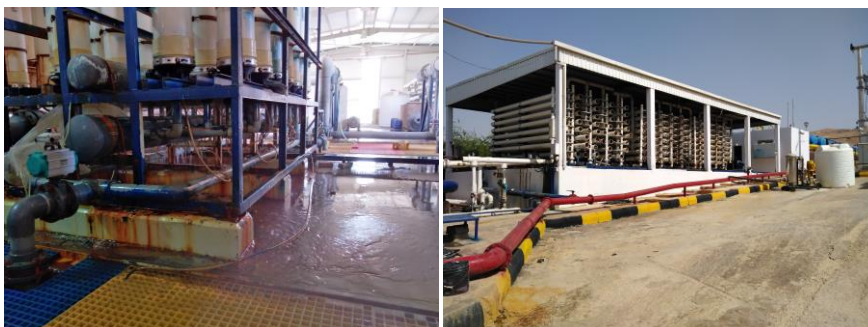
Left: The project will support improving the KEMAPCO desalination plant operated by AquaTreat for water supply to Aqaba.
