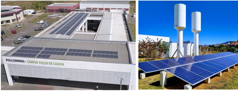
Photos 3 and 4: Solar panel installations at the Federal Institute (IF) - South of Minas Gerais and Poços de Caldas, Brazil
