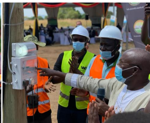
Photo left: Installation of solar panels in one of the villages benefiting from the installation of 40 solar mini grids in Northern and Southern Uganda © GIZ PREEEP
