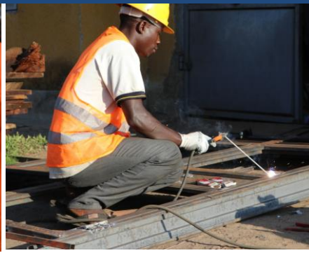
Photo left: Solar trainees during a practical session at the Renewable Energy Training Centre based at Nakawa Vocational Training Institute. © GIZ PREEEP
