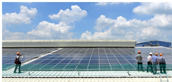
Rooftop solar at a factory in Southern Viet Nam. Photo: © GIZ
