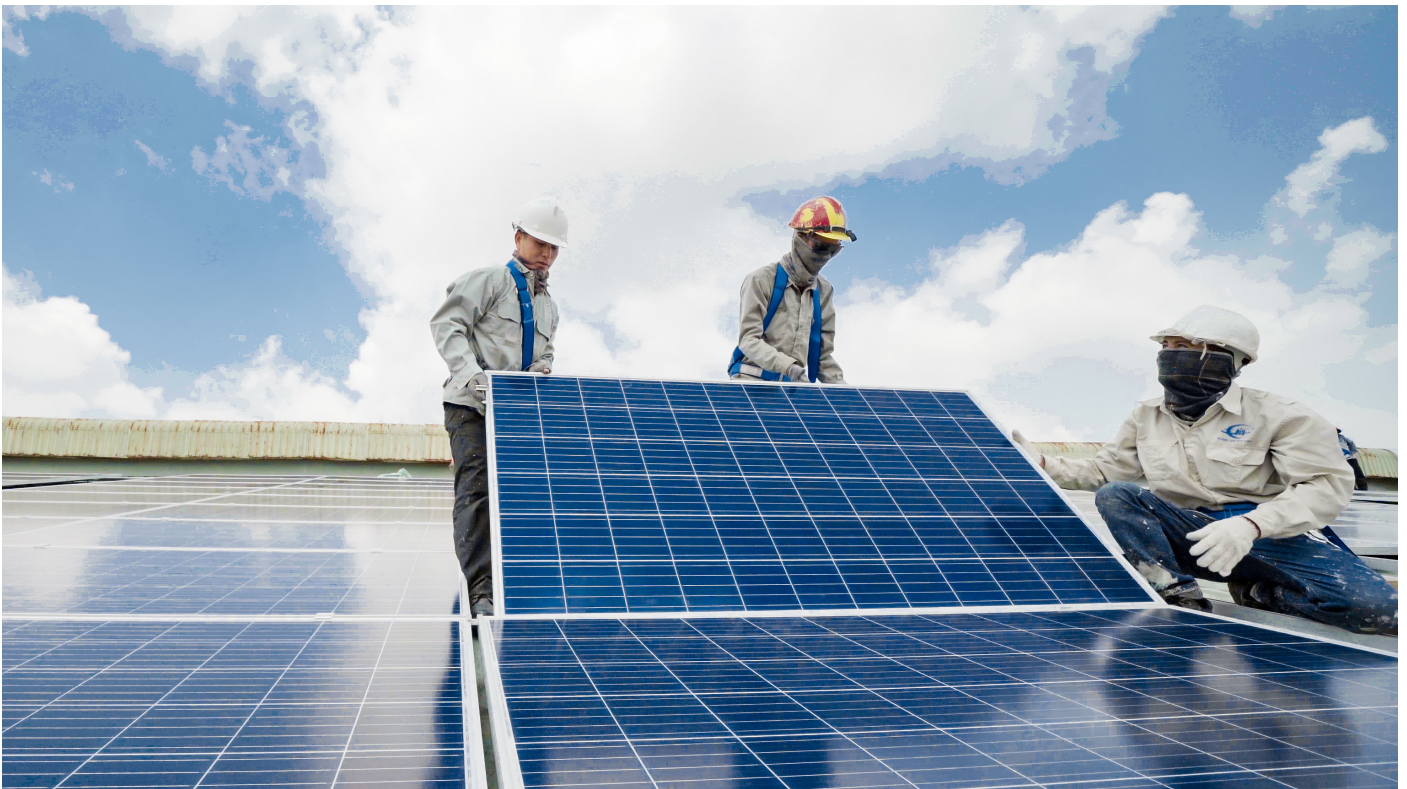
Rooftop solar at a factory in Southern Viet Nam. Photo: © GIZ
