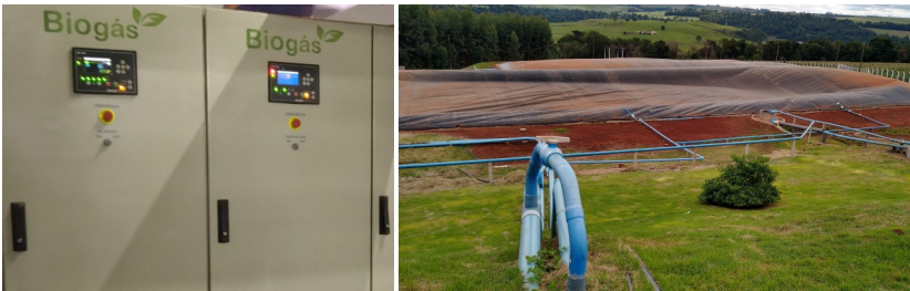
Photos 3 and 4: Biogas production in Toledo (PR).
