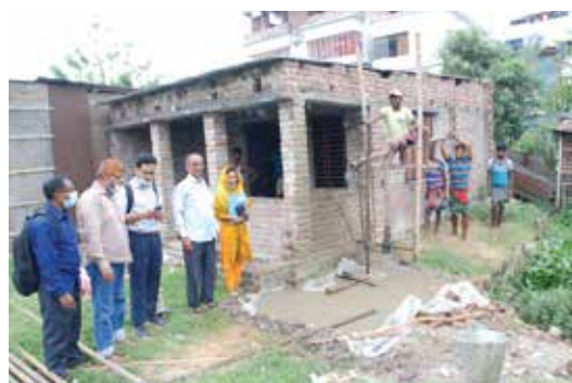
With the financial support of a charitable person, the submersible pump is being installed for safe drinking water at Court Station Slum, RCC
