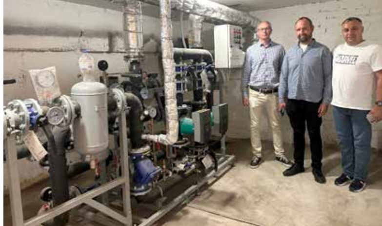
Individual heat substation installed in a multi-apartment building under “Energodim” programme in Svitlovodsk city.
