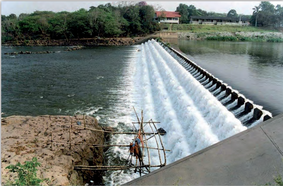
Figure 74: A weir oxygenates water downstream of Ubolratana Reservoir, Nam Pong River, Thailand
