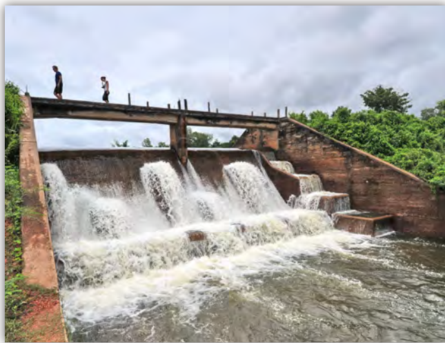
Figure 22: A simple pool-and-weir fish pass (right background) at the Huay Siet Weir in Lao PDR
