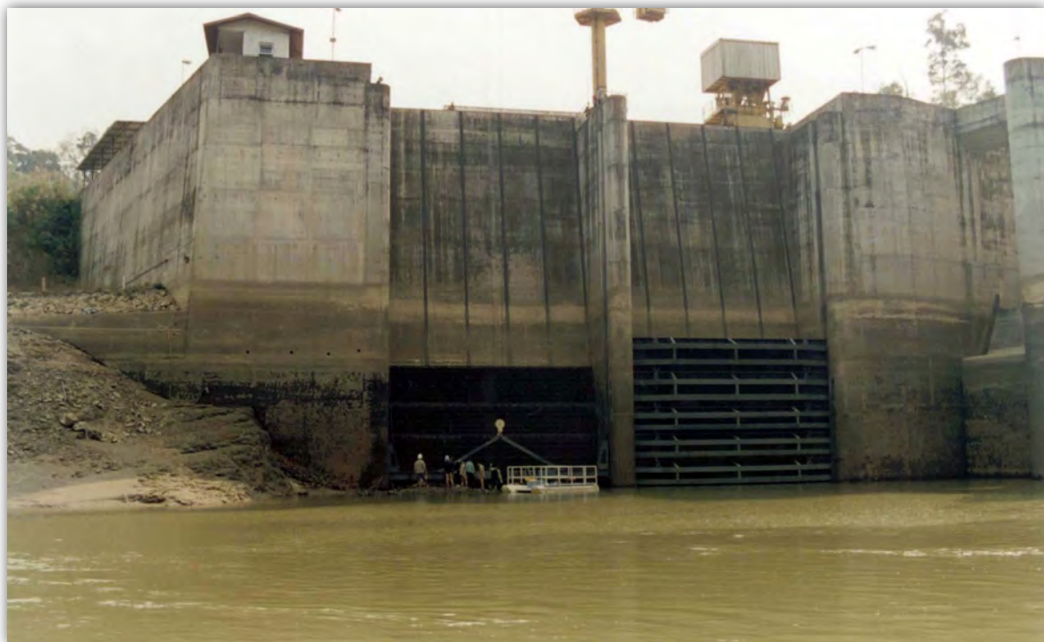
Figure 51: Large screens on the intakes of the Theun-Hinboun hydropower plant in Lao PDR in 2001.
