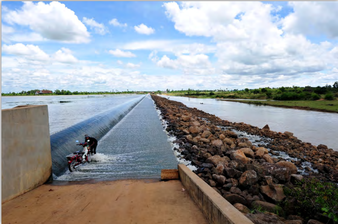
Figure 10: Spillway of Stung Chinit, a large shallow irrigation reservoir in Cambodia Photo: Kent Hortle
