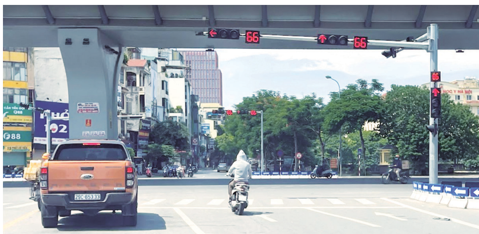
Figure 6.4. Near-sided bicycle signals improve the sight distance of bicycle users at intersections
