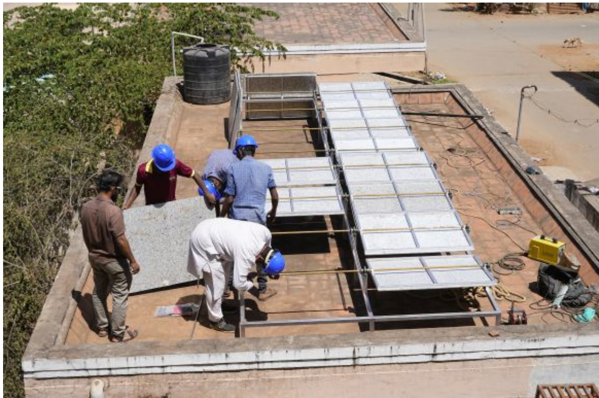
The Alufoil blinds are installed on the roof to keep the building cooler during the hot days © GIZ
