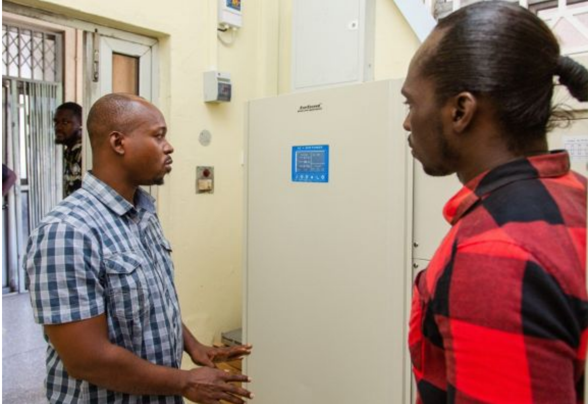
The GIZ team is shown the voltage stabilisers installed in the server room by hospital technicians © GIZ
