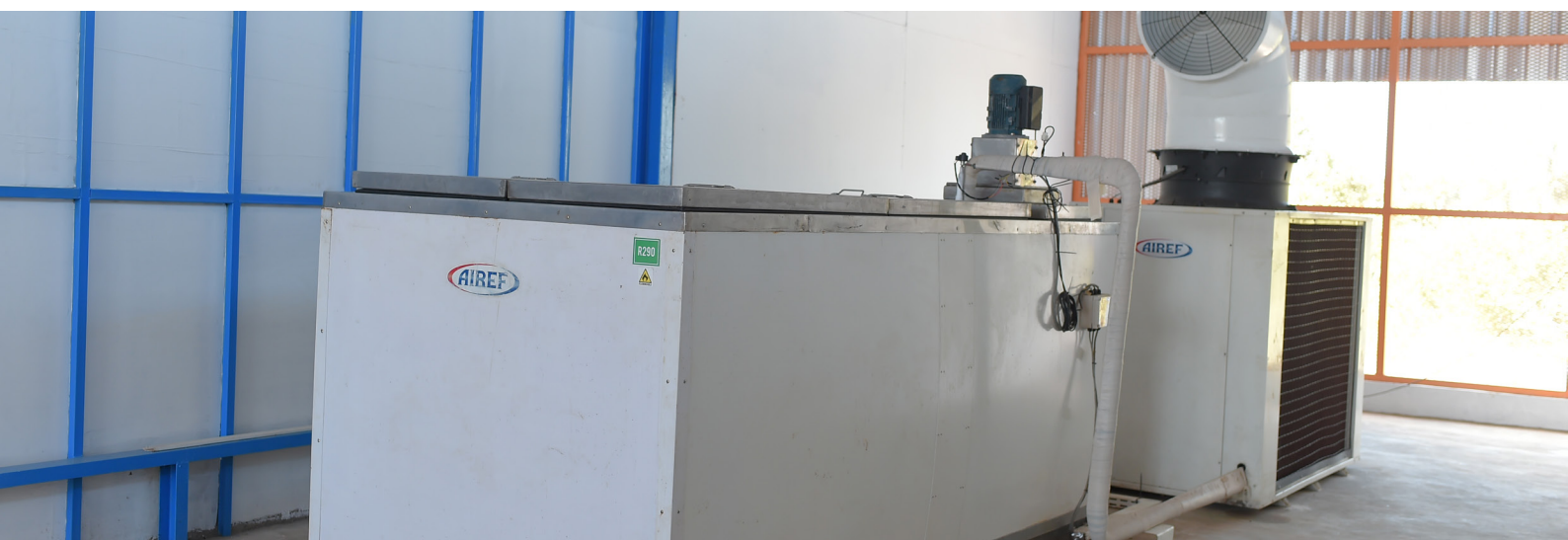
FIGURE 3 | Integrated cooling system of the Solar Ice Maker, Sulamu, installed within the facility.
