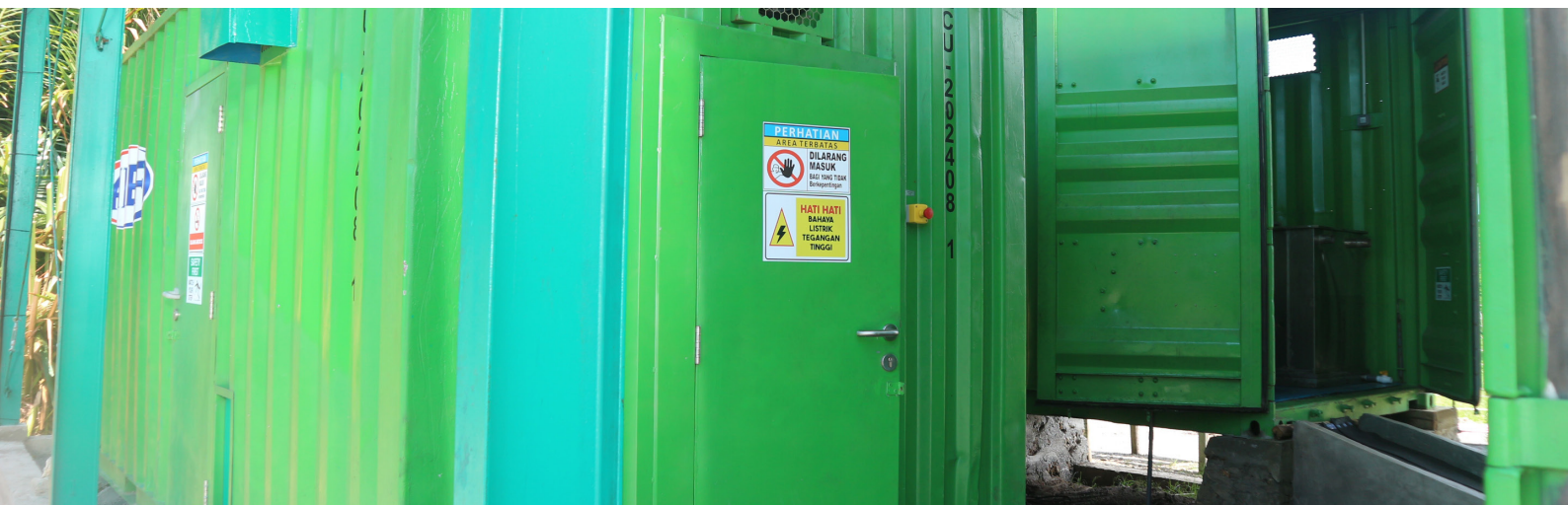
FIGURE 5 | Modular container-based design of the Solar Ice Maker in Kawa, comprising three interconnected units.
