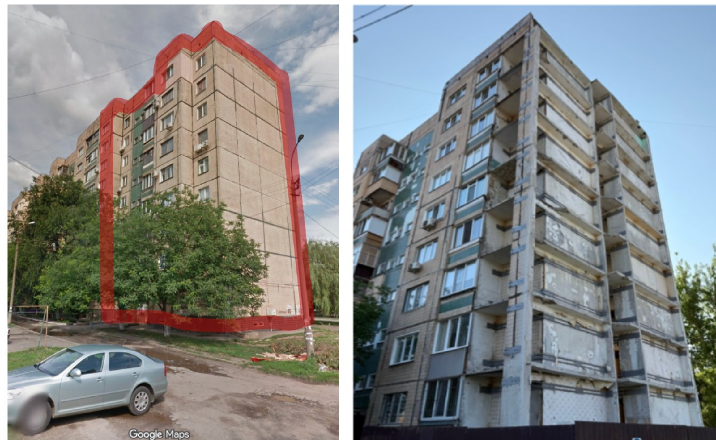
Kryvyi Rih Pilot Building No.1, Українська,55 A typical multi-family 9-storey Initial assessment indicated the need for façade repair, energy retrofitting, and partial structural intervention.
