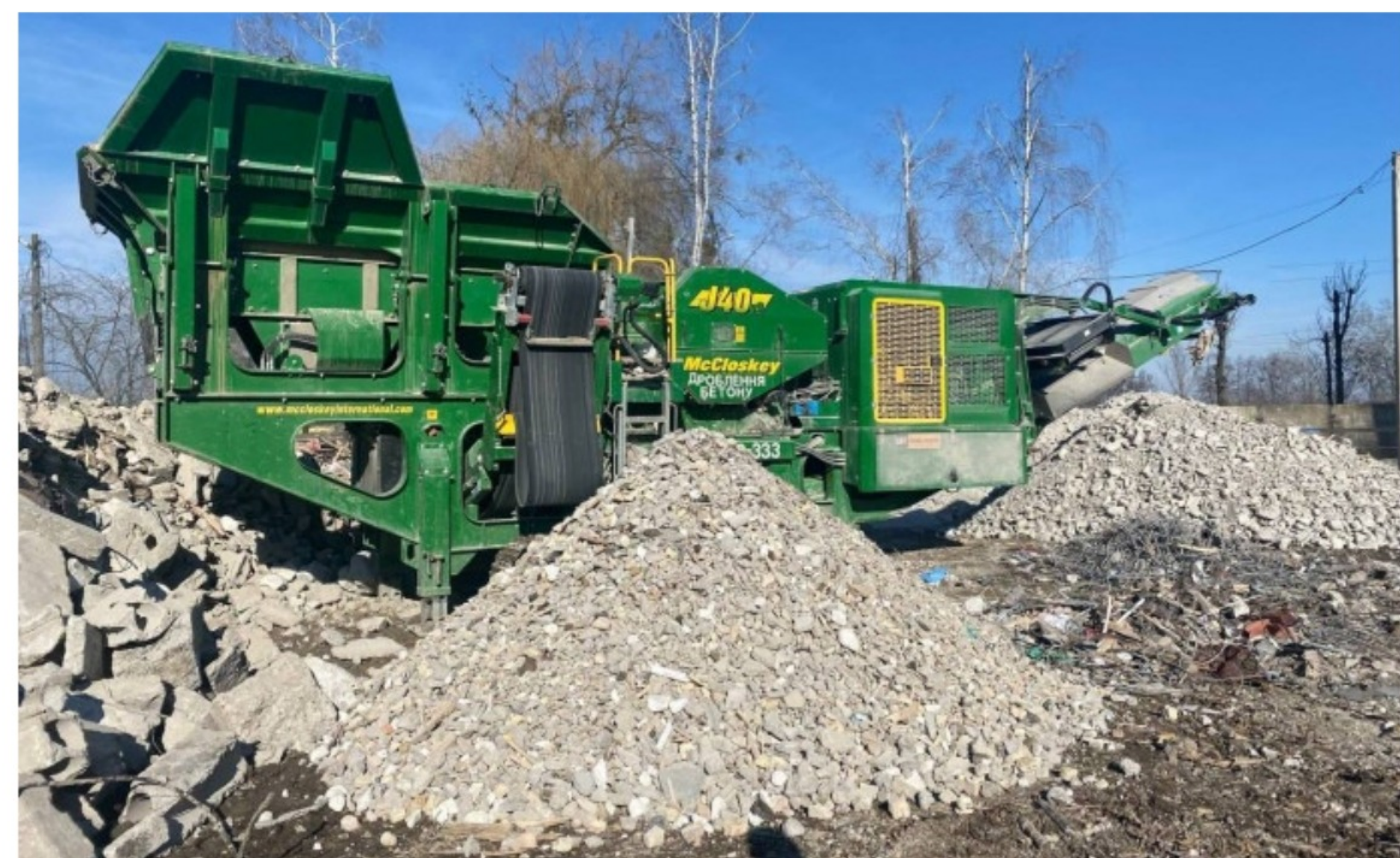
The process of crushing construction waste and turning it into new building material © Neo-eco
