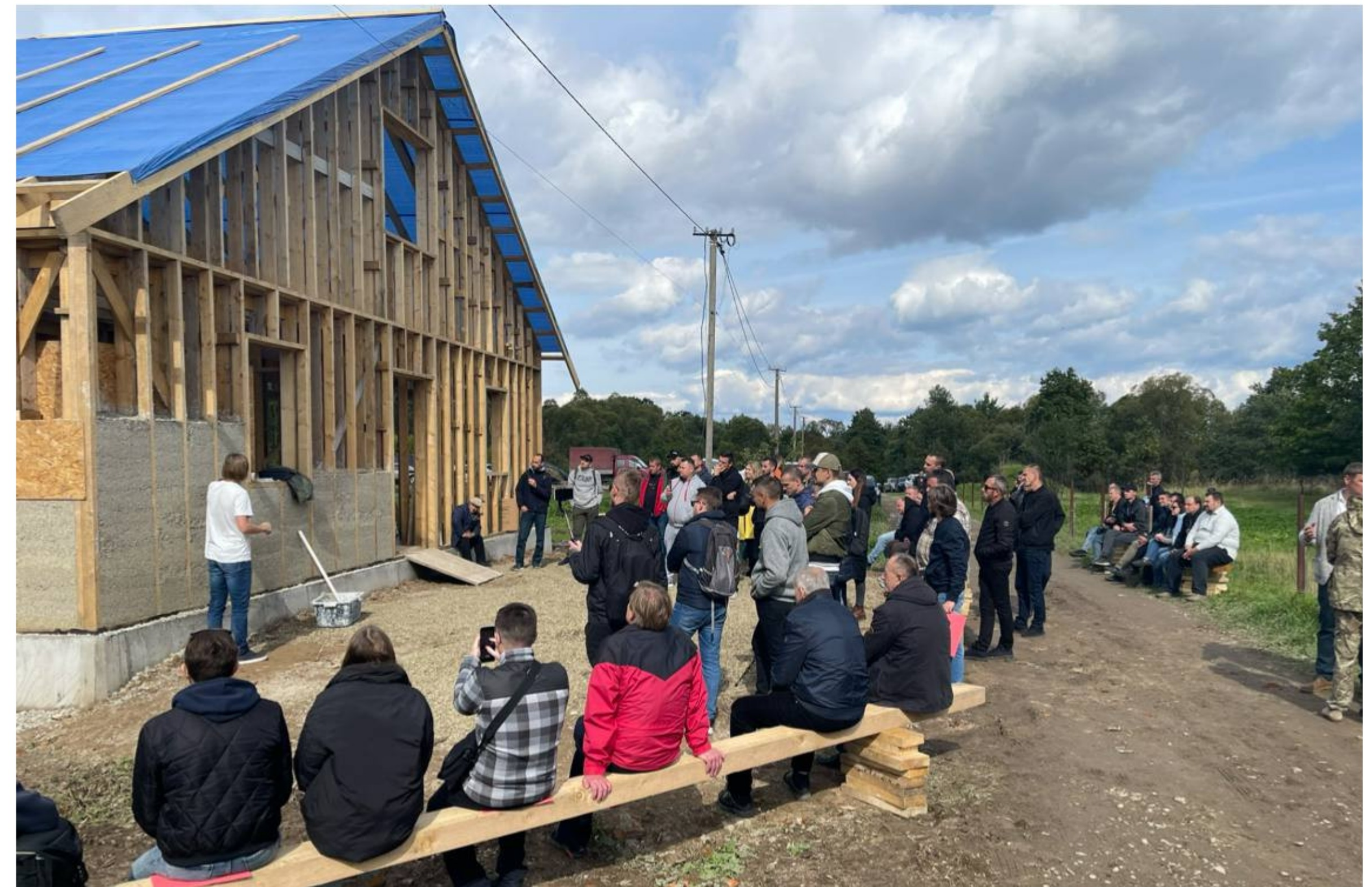
Construction of eco-friendly housing for refugees using Hempire™ (hempcrete) technology while training internally displaced persons in this technology.
