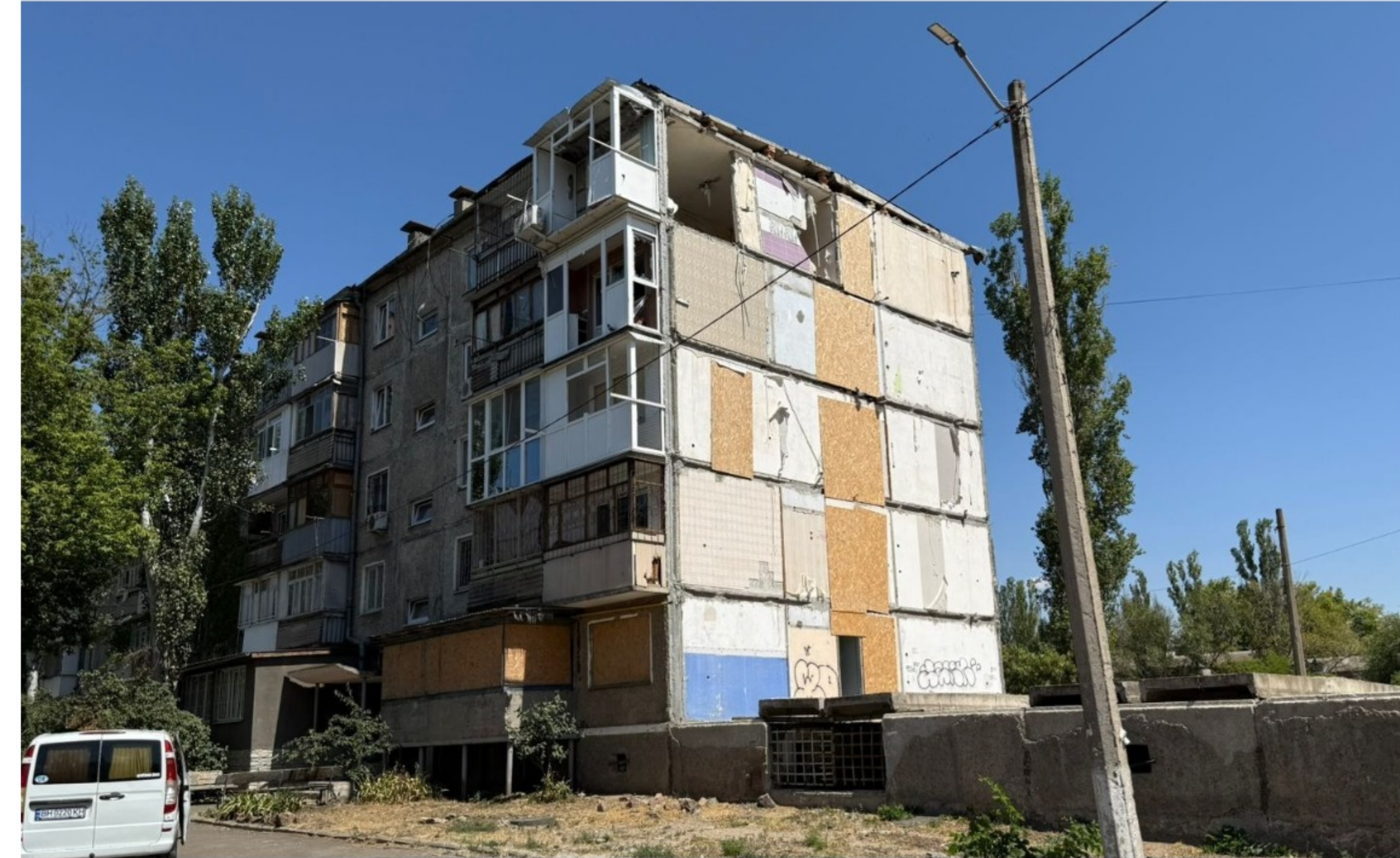
Mykolaiv Pilot Building 49/1 General Karpenko Street A representative 5-storey panel residential building It belongs to one of the most widespread 1960s housing series found across Ukraine’s cities and district centres.
