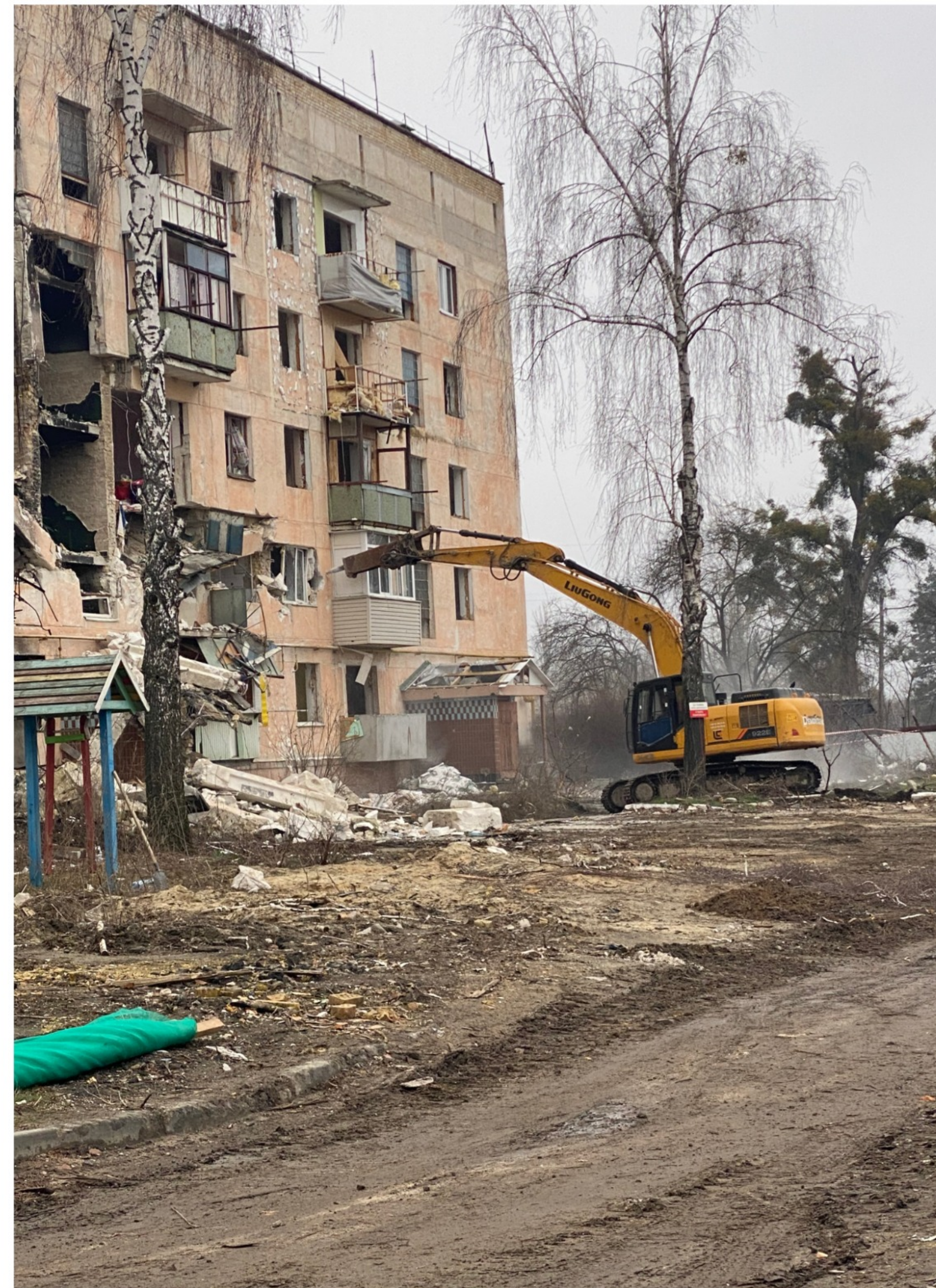
Neo-Eco Ukraine is dismantling a damaged high-rise building in Gostomel. Photo provided by the company.
